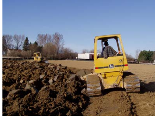
Soil corrections underway on an EDA owned lot in the industrial park.
