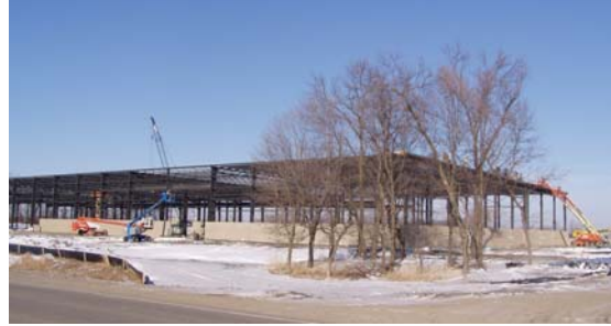
Construction began on Warrior's new 92,000 square foot production facility in the fall of 2006.
